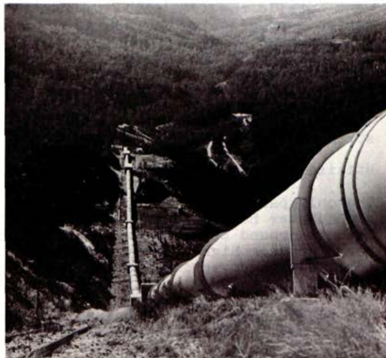
Pipeline down West Kiewa valley conducts water for the generation of electricity.
