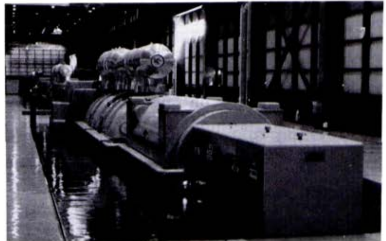
Inside the generating room of a power station
