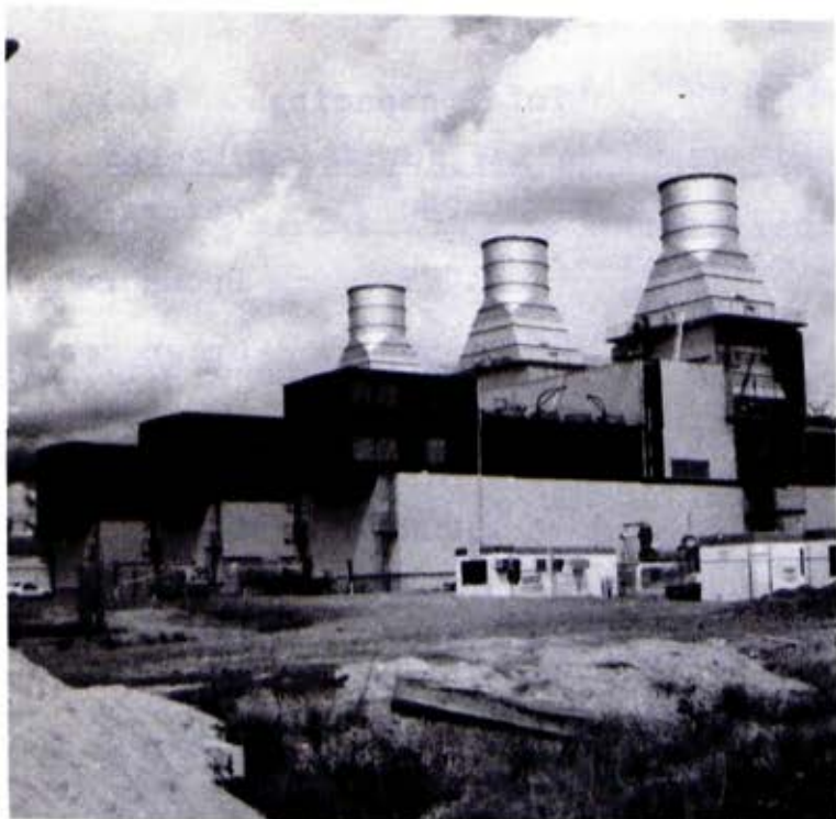
Gas turbine generators with a capacity of 225 MW located north of Jeeralang
