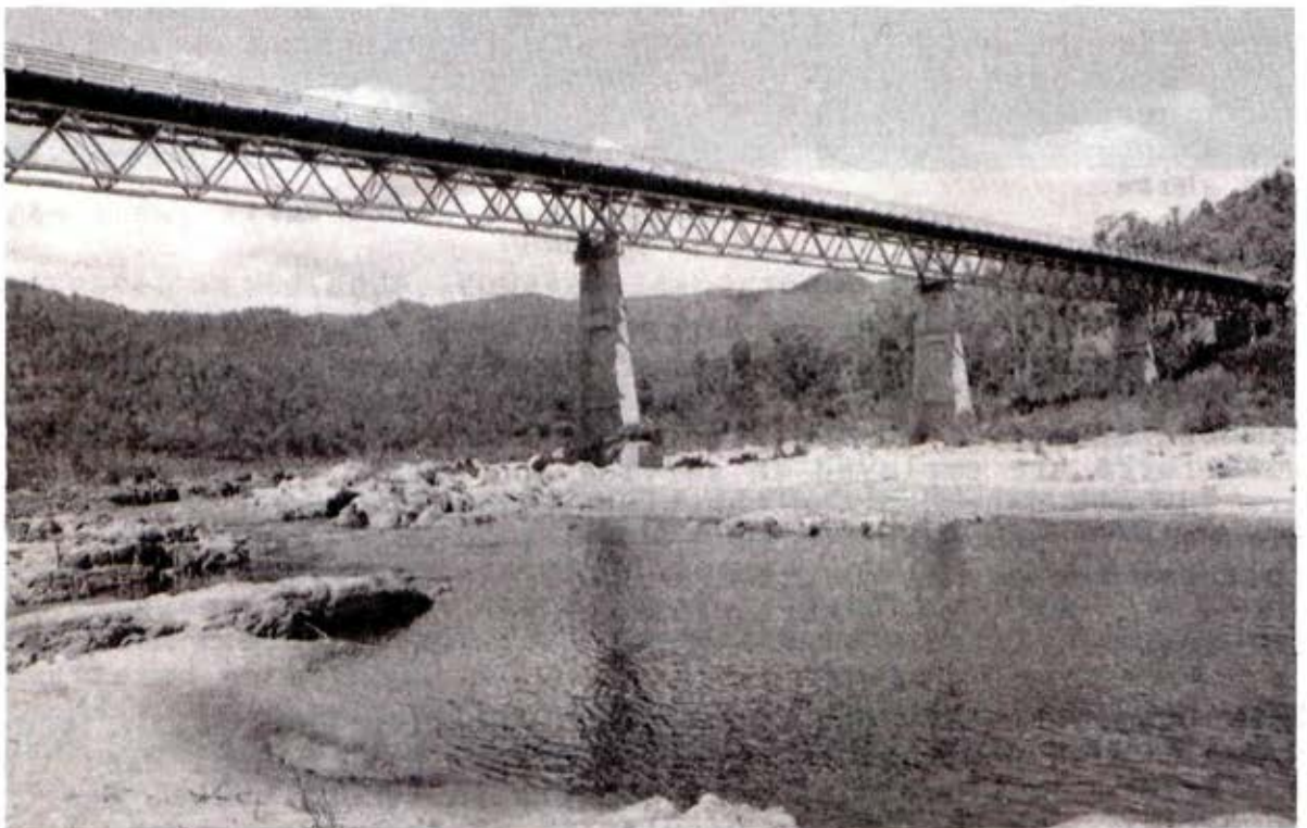
The MacKillop Bridge, the only road crossing over the Snowy River between Orbost and the border
