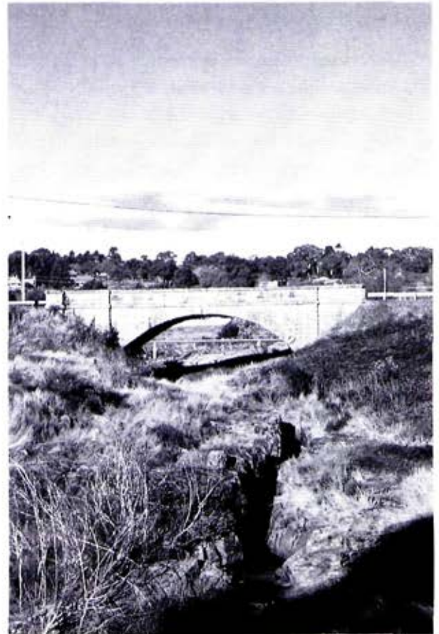
Single catenary arch road bridge constructed of local granite in the goldrush era, Beechworth.
